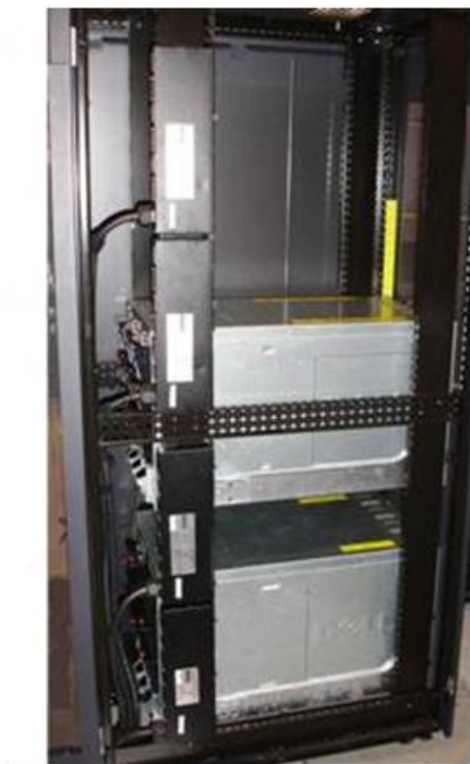
Figure 5 – Mounting of four PDUs in the 0-U Space of the Dell 4210 Rack.
