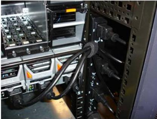
Figure 2 – The 24 Amp Three-Phase PDU connected to Power Supply Units. The 48 Amp Single-Phase PDU (not shown) is connected in the same manner. Note that the jumper power cords are secured to the system strain relief bar.
